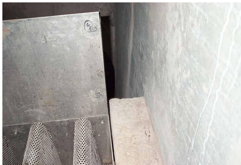
Photograph 3 – Unscreened Flow Bypass due to poor Installation
