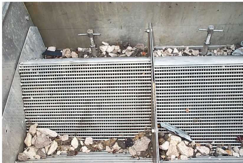
Photograph 4 – Construction Debris left on top of Screen
